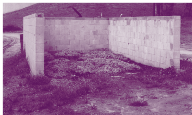
A structure such as this concrete block bin can store manure accumulated over many months. Ideally the storage should be covered to prevent groundwater and surface water contaminations.
